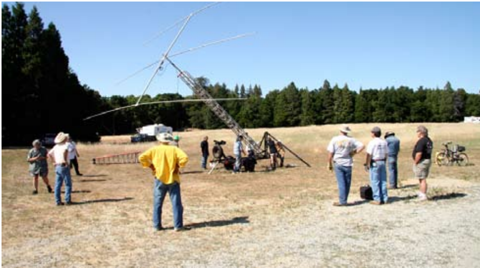
Installation teams raise the tri-band Yagi antenna in preparation for Field Day operation Photo by: Rich Seifert, KE1B
